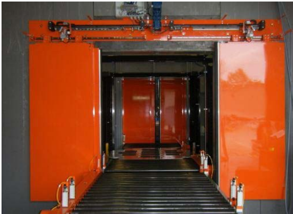
Lead primary shield vault
