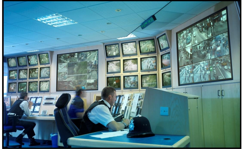
Typical operator control room
